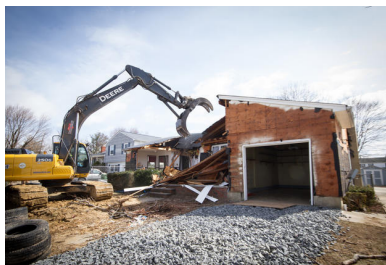
The first house to be demolished as part of the Blue Acres buyout program, in Sayreville, NJ in March 2014. Photo courtesy: Rosanna Arias/FEMA
